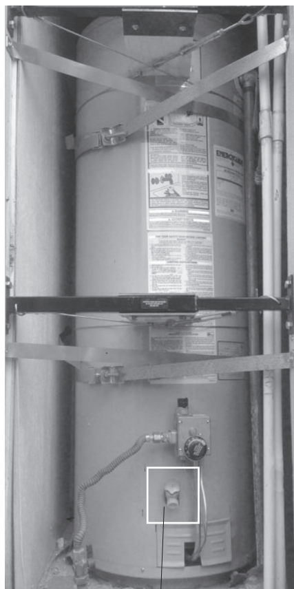
Hot water heater faucet
