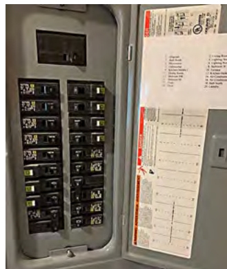
Breaker box open
